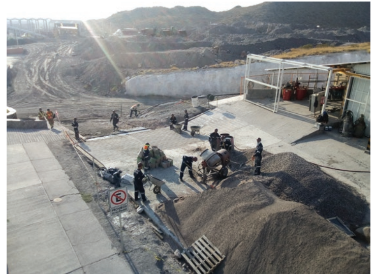
Workers installing a new concrete pad outside of the Platosa surface maintenance shop
