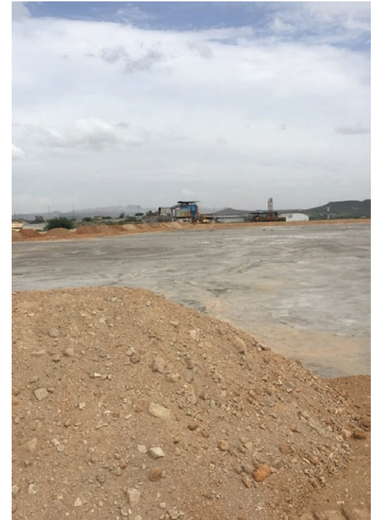
Soil stockpiled to complete covering of the decommissioned TMF #1 at Miguel Auza
